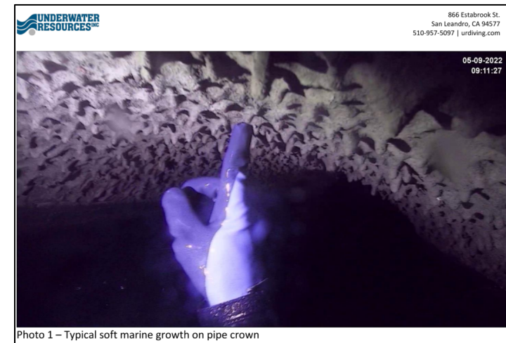
Photo 1 – Typical soft marine growth on pipe crown
