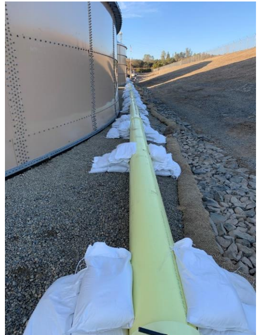
Figure 4. project photo courtesy of San Juan Water District showing above-ground pipeline installed.
