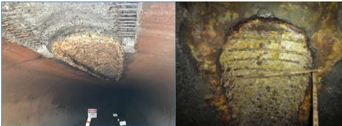
Photo 2: Concrete and rebars exhibited severe corrosion for 96-inch and 87x136-inch pipelines
