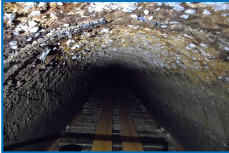
Figure 1. EBMUD South Interceptor showing severe corrosion
