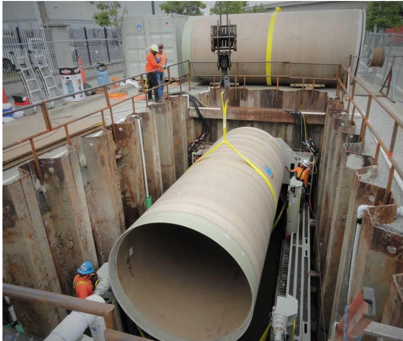
Figure 6. New pipe being lowered into pit, and next pipe ready to be lowered
