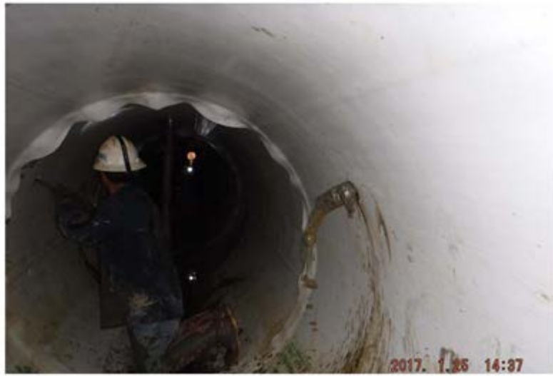
Figure 10: Tunnel Grout Port (Photo by Staheli Trenchless)
