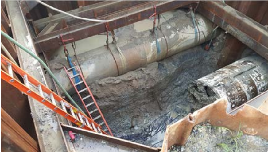
Figure 11: Tunnel Machine Exiting the Receiving Pit (Photo by City of Redwood City)
