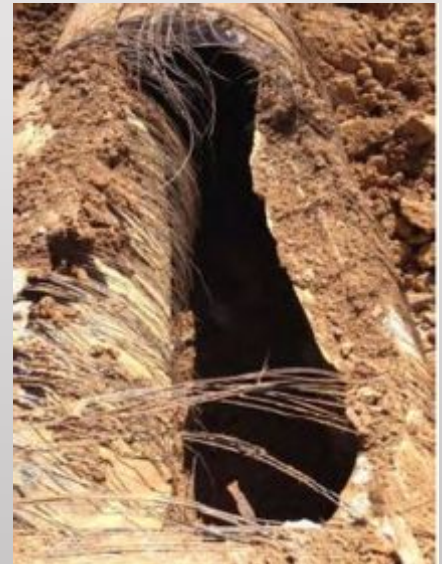
Ruptured pipe visible after water subsided
