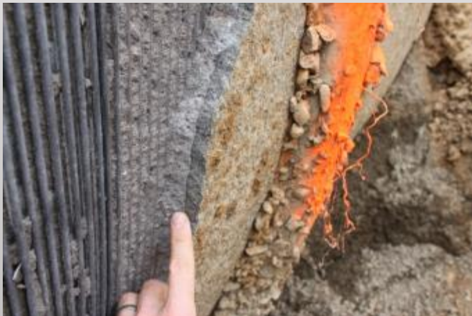
Layered mortar coating near downstream joint. Outer layer applied as a local patch.
