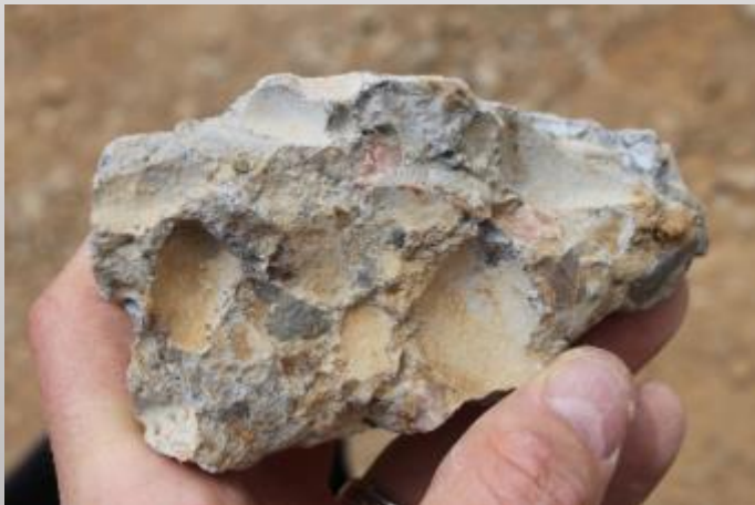
Aggregate pullout in concrete core
