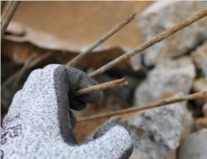
Brittle wire fracture surface
