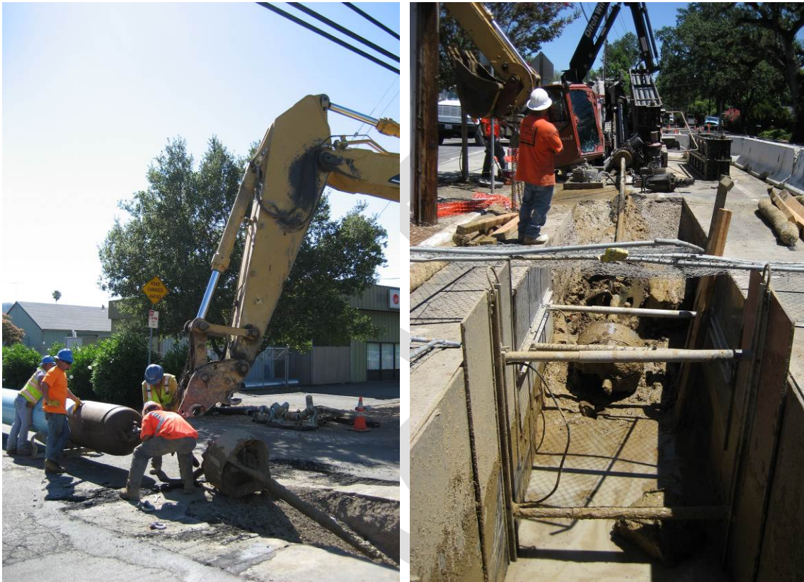
Figure 2. Installation at Salvador Avenue avoiding the overhead utilities during pullback from the exit pit on the west side of Hwy 29 (left) to the restricted receiving pit on the east side of Hwy 29 (right).
