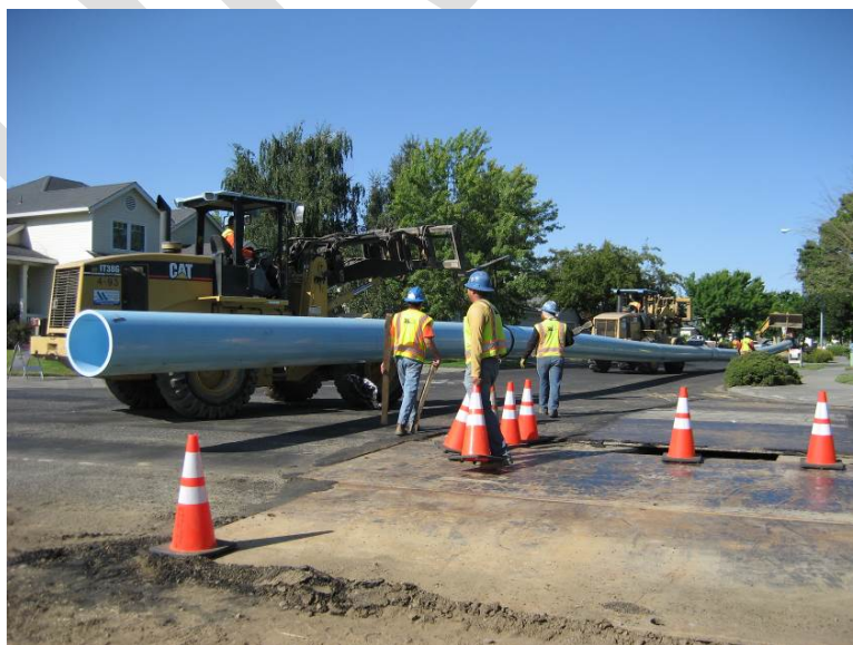
Figure 4. Installation procedure shown for the Sierra Avenue crossing required moving sections of fused pipe,
