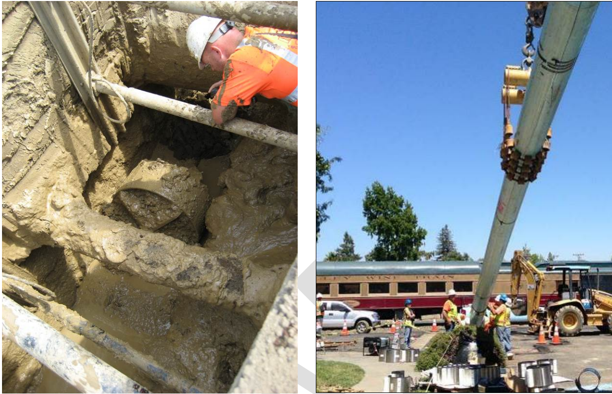
Figure 5. Challenging components of the Sierra Avenue crossing included working within close proximity of high pressure gas and water transmission mains (left), and underneath the Napa Valley Wine Train (right).
