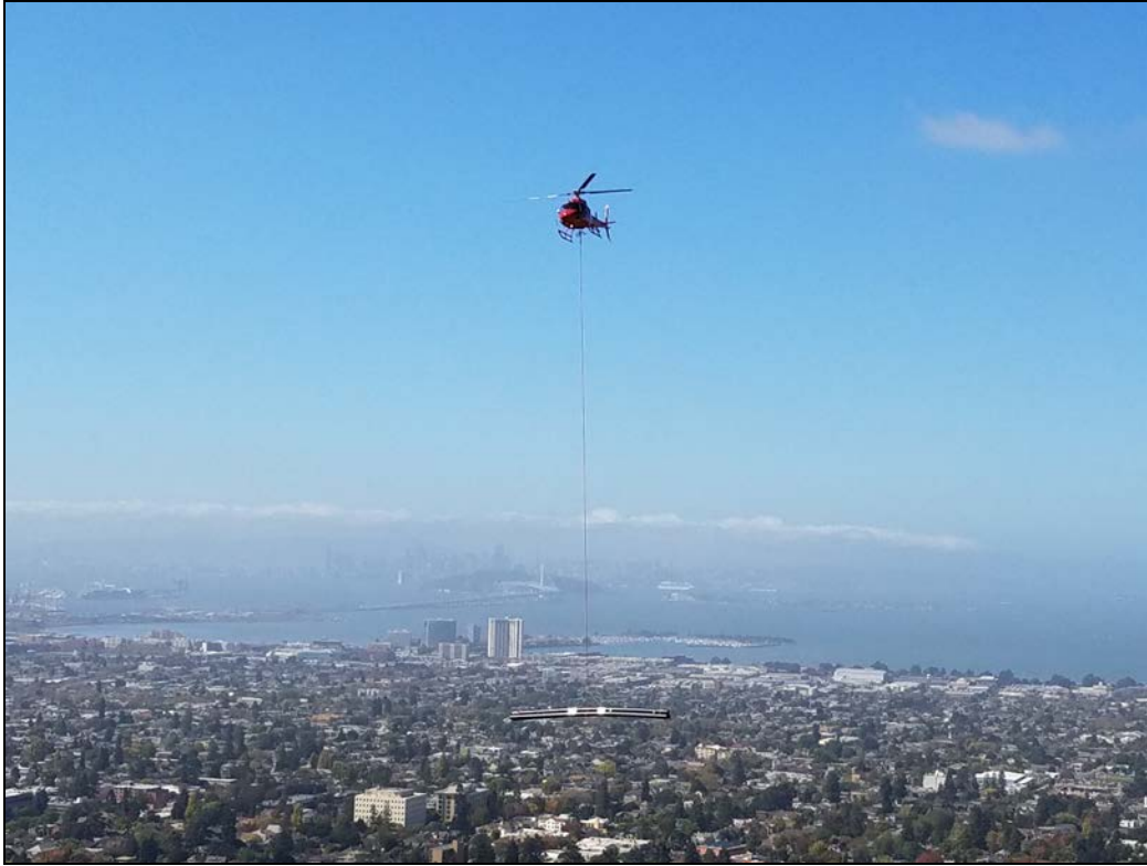
Figure 4. Helicopter Delivering Bundle of HDPE Pipe for the Panoramic Hill Pipeline Replacement Project
