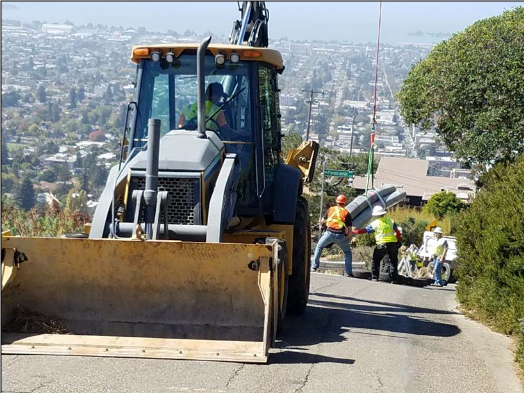
Figure 5. Airlift Delivery Location on Panoramic Way for the Panoramic Hill Pipeline Replacement Project
