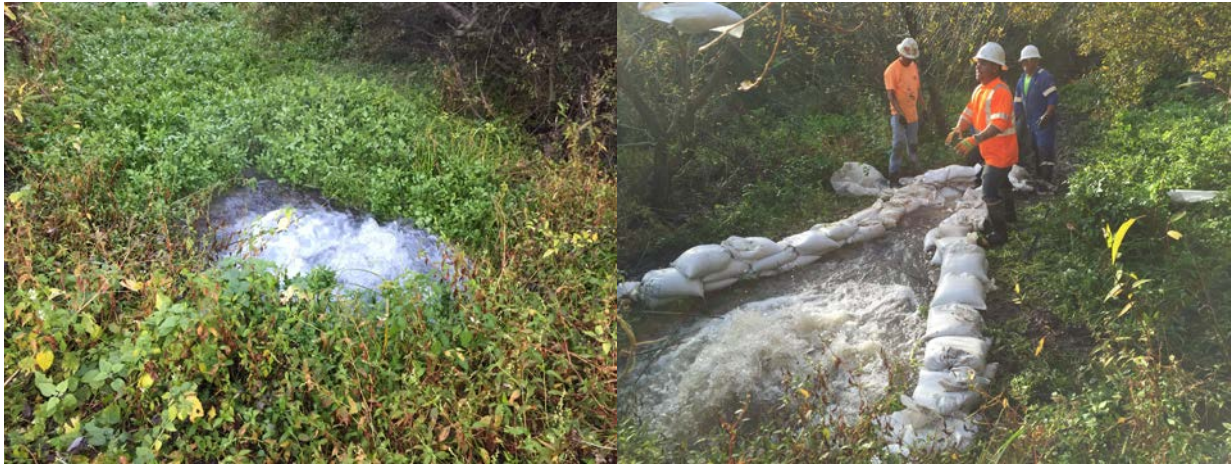
Figure 3: Ruptured water main.
