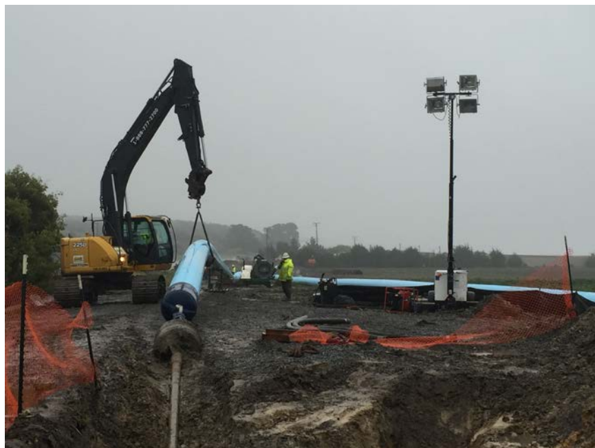
Figure 9: Commencement of Pullback of the 30-in. Barrel followed by the 24-in. Pull-head and 24-in. FPVC.
