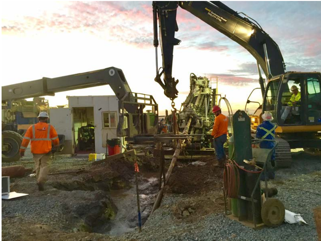
Figure 8: American Augers Rig with 380,000-Pound Thrust and Pullback Capacity. Reamer at Entry Pit.
